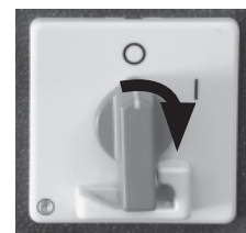
Switching on the power switch
